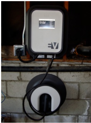
Sedan's charger, in garage.
